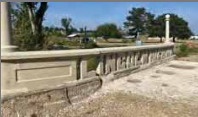
North side of the Lincoln Highway Bridge on August 21, 2023 Photo by Mary Helen Preston
